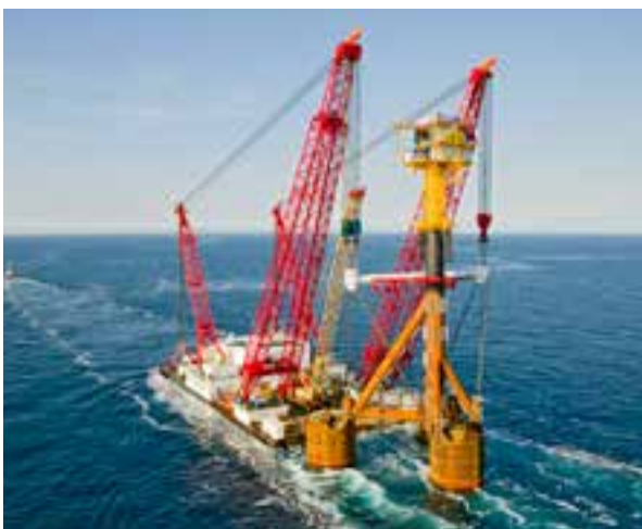
L6-B platform in the hooks (picture courtesy of Wintershall Noordzee B.V./Scaldis)
